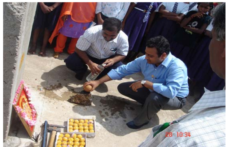
President Rtn Rahul Aggarwal inaugurating the construction of Science Lab and Class Room.
